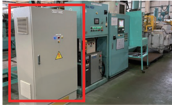
The equipment was installed between the control panel of the casting machine and the hydraulic pump motor.
