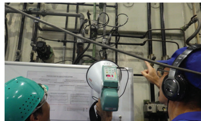
Diagnosing the air leaks
